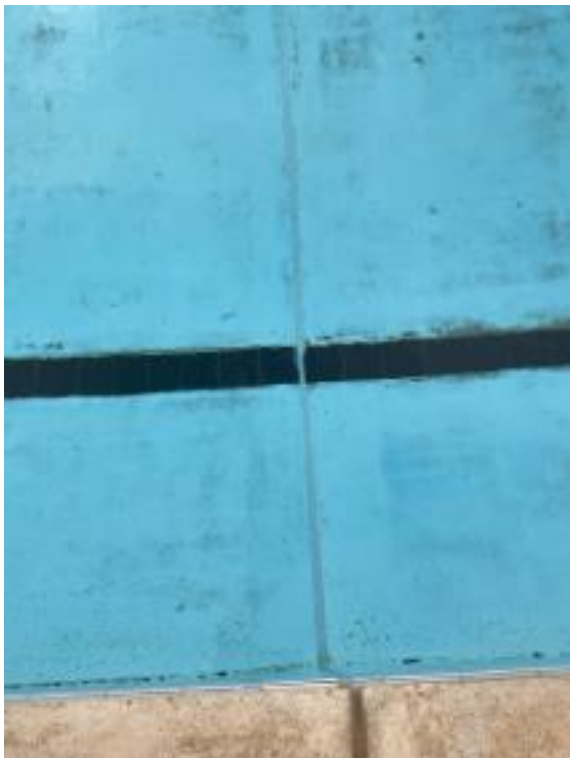
Different width of the expansion joint sealant
