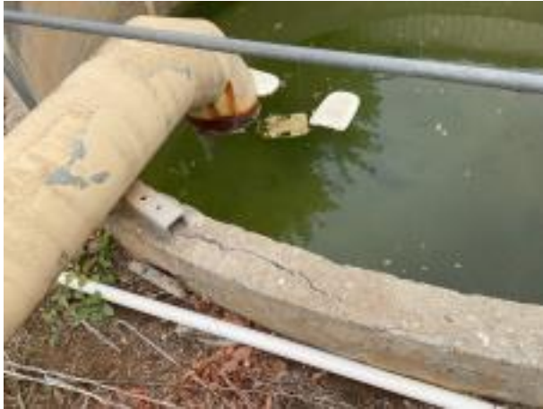
Damaged Balance Tank wall, rusted pipe and rubbish
