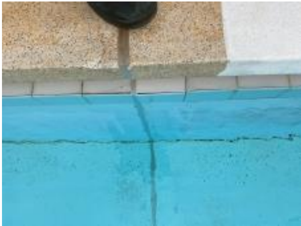
Cracked and debonded tile
