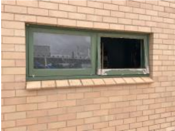
Broken window in Plant Room
