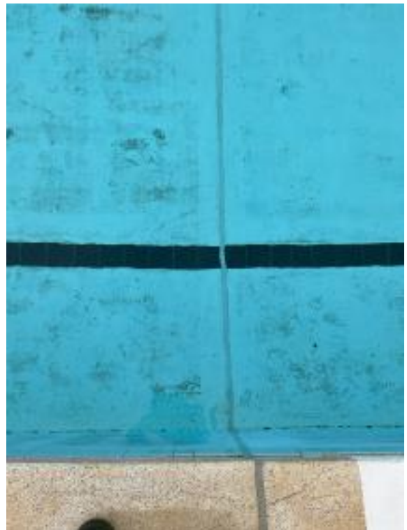
Cracking in the pool floor
