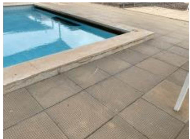
Concrete upstand cracking
