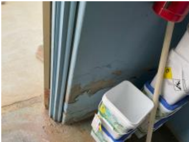
Plant Room wall damaged by chemicals
