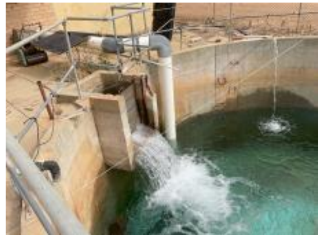
Damaged Balance Tank
