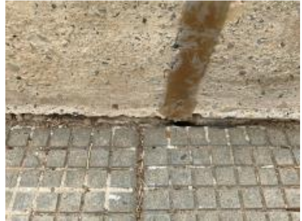
Settlement of the concourse
