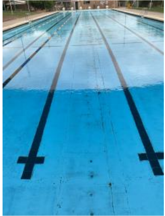
Cracking along centre line
