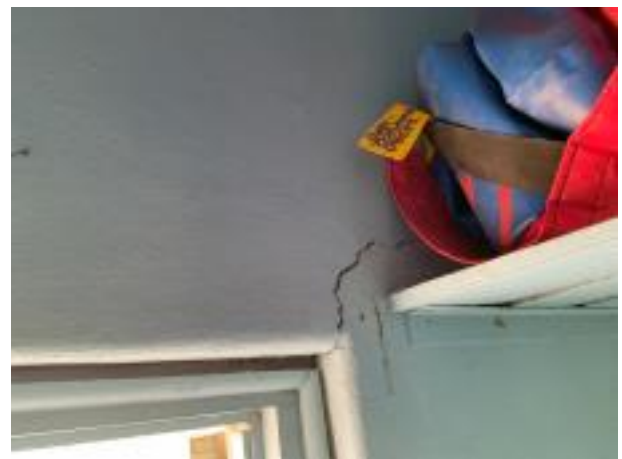
Structural crack above Plant Room door
