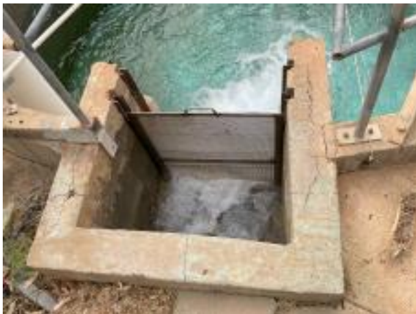
Broken strainer screen (Balance Tank)
