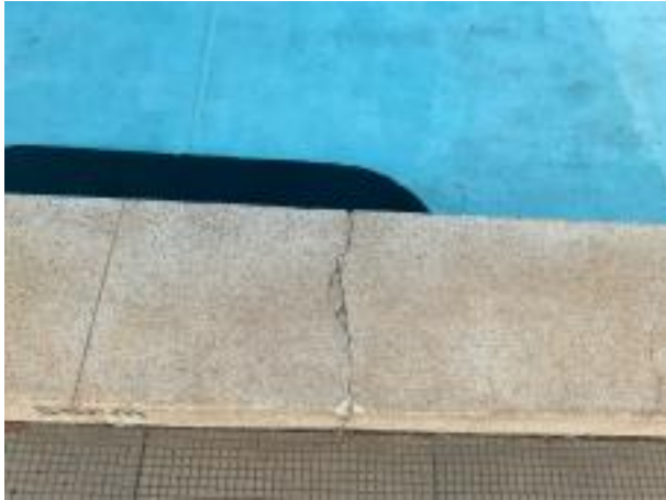
Concrete upstand cracking (no handrail)
