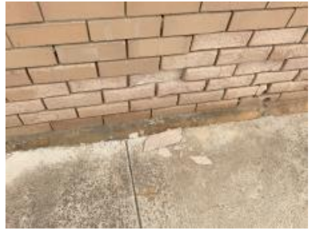
Spalled brick and lost damaged mortar
