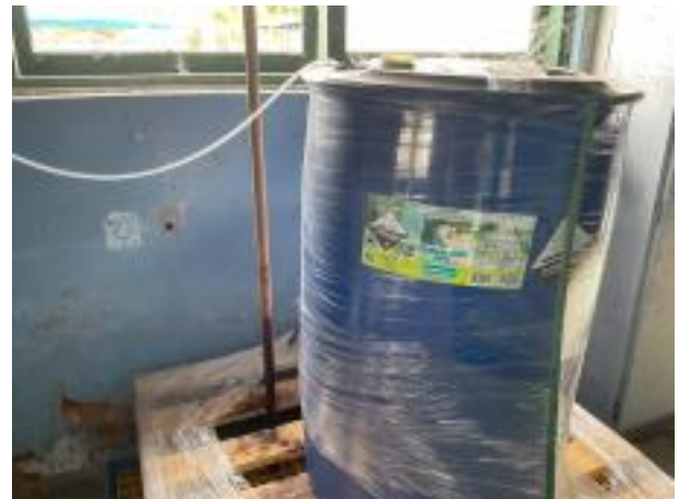
Sulfuric Acid - pH regulator
