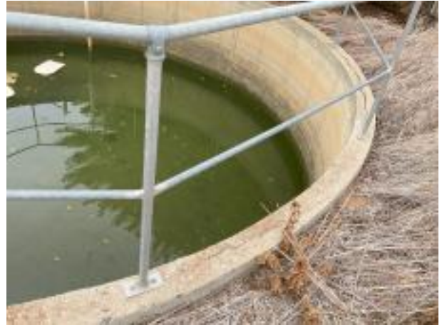
Cracked wall and unsafe balustrade
