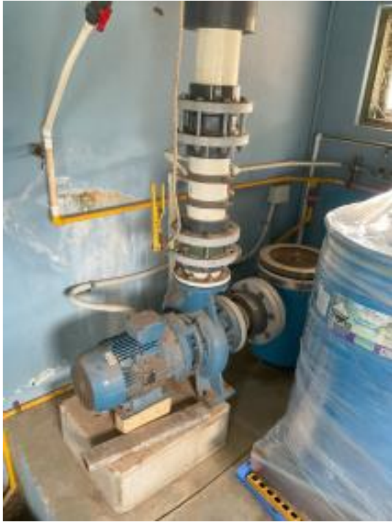
Insufficient pump fixing
