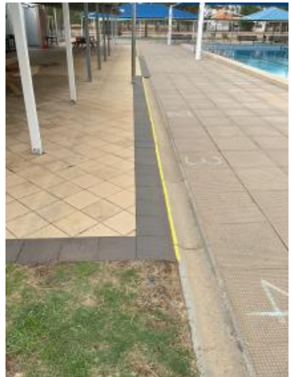
Concourse drainage channel – trip hazard
