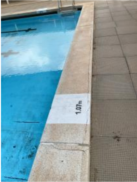
Cracking in the concrete upstand
