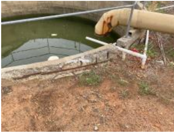
Spalled concrete wall and rusted reinforcement
