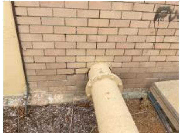
Damaged mortar around the pipe
