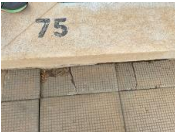
Concourse cracks and settlement
