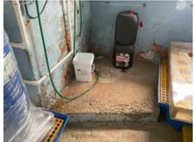
Degradated concrete plinth and brick wall
