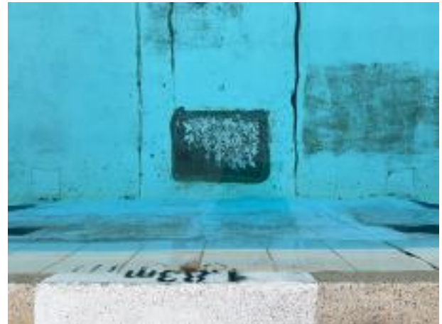
Concrete patches at deep end
