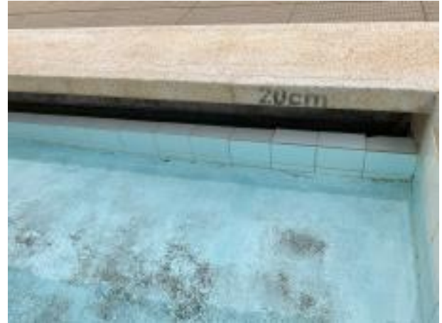
Debonded tiles and concrete upstand cracks
