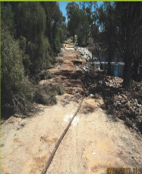
Storm damage – Mackie Siding Road
