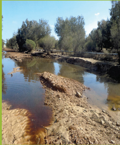
Storm damage – Duck Pool Road
